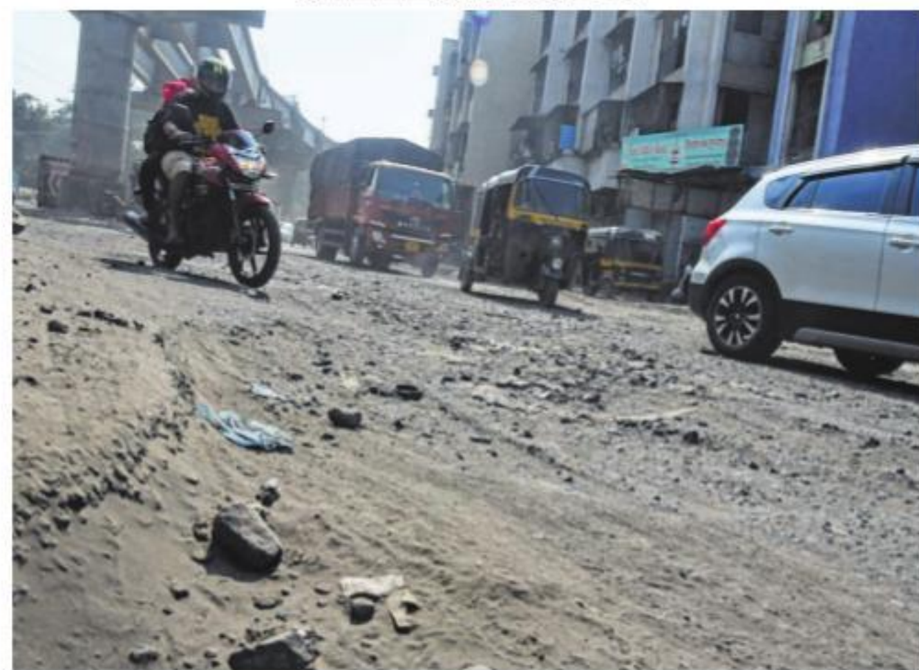
The roads from Kasheli to Anjurphata (in Thane) have deteriorated, increasing the risk of accidents and raising concerns of respiratory diseases caused by unsettled dust. PIC: VIBHAV BIRWATKAR
