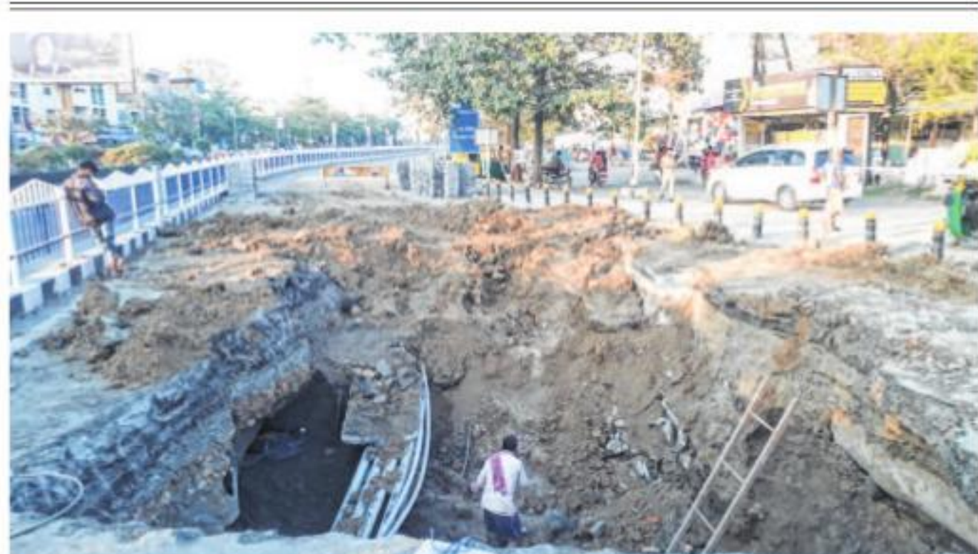
Due to IMC sewerage line work at Vijay Nagar Square, the traffic has been diverted on the BRTS lane causing trouble to commuters as well as i-BUS which also takes the same route increasing risk of accident. PIC BY - PINTU NAMDEV
